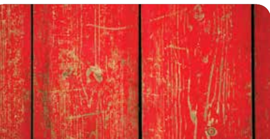
STABILIZE WOOD THAT HAS BECOME CRACKED OR DAMAGED
